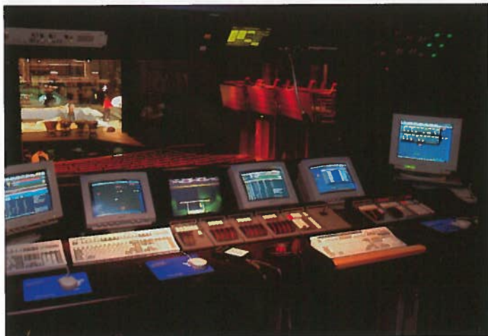
The lighting control set-up. To the left of the video monitor there are additional two work stations for work with the system on- and off-line.
