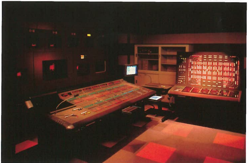
The custom Aviator console and geographic patch bay at Tokyo Broadcasting System's studios - the installation is identical in Studios A and B, apart from patch layout.
